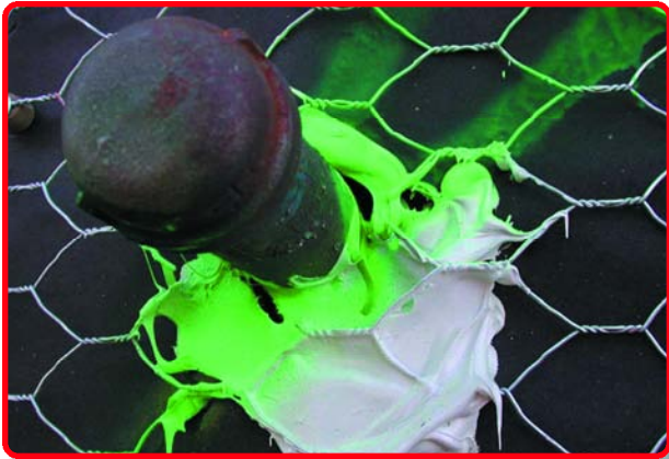
Plumbing Gas Pipe with Caulking
