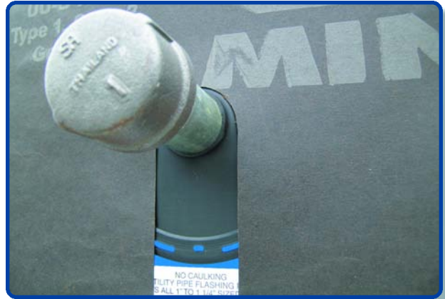
Plumbing Gas Pipe with QF Flashing Panel
