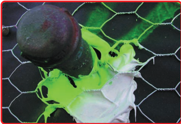
Plumbing Gas Pipe with Caulking
