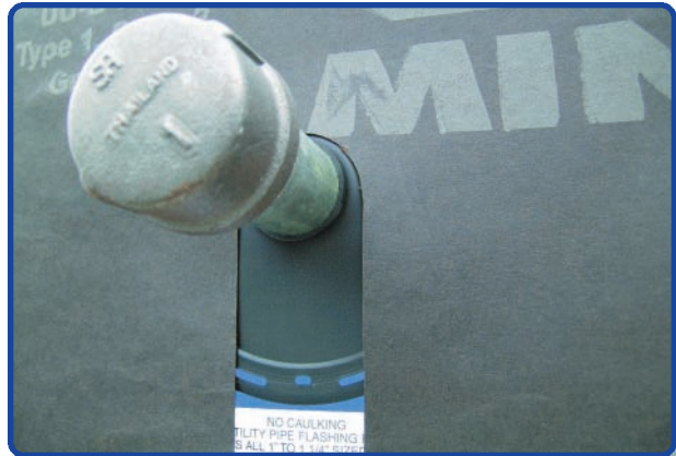
Plumbing Gas Pipe with QF Flashing Panel
