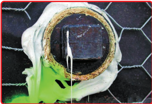
Plumbing Clean Out with Caulking
